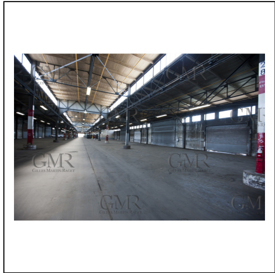
07/06/2011 - San Francisco (USA,CA) - 34th America's Cup - The Piers in their state of origin - Pier 23
